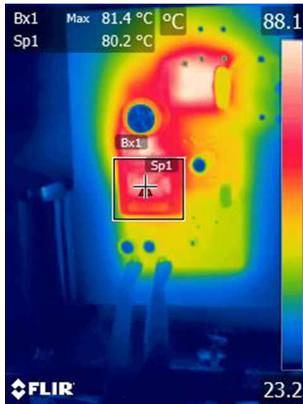
Figure 2-7. Front of the Board – Transformer Showing 80°C
