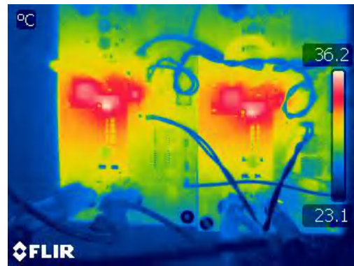
Figure 4-24. Thermal Condition in Dual Phase Boost ( V_{IN}=15V and 2A Load)
