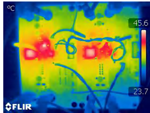
Figure 4-32. Thermal Condition in Dual Phase Buck ( V_{IN}=30V and 2A Load)
